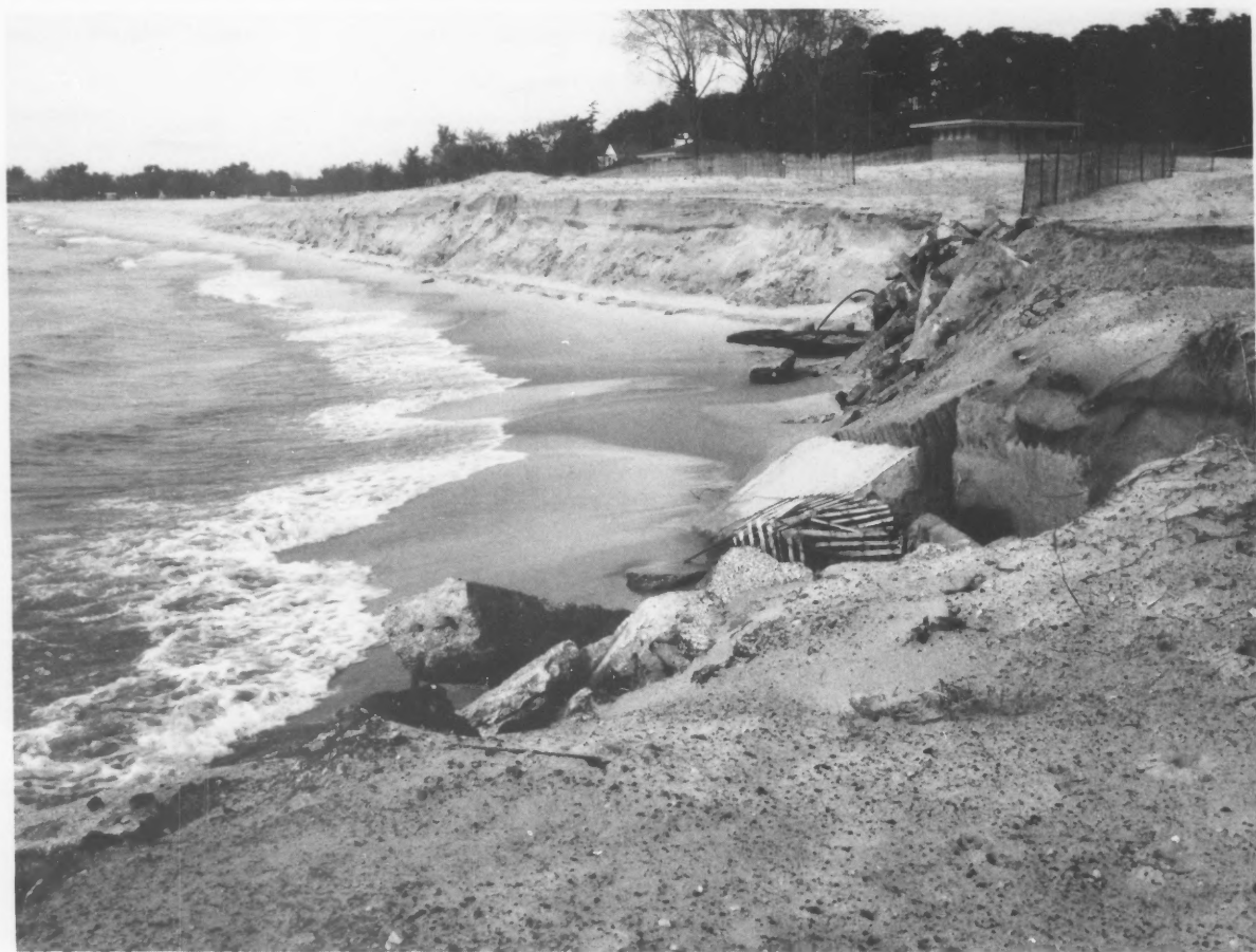
Fierce Lake Michigan wave action undermined these sand dunes and beaches at South Muskegon, Michigan. To help break up the wave action, boulders have been placed at several locations.
