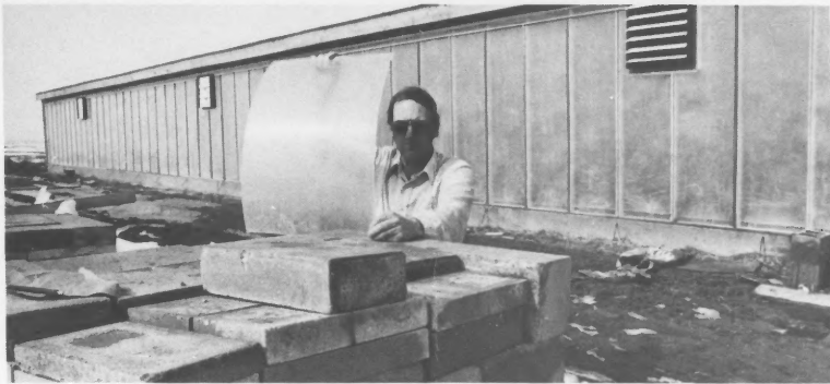
Dale Keesecker's solar collectors were built from concrete blocks and resin reinforced fiberglass panels. All materials needed to build a solar-powered farrowing house are readily available to producers through building contractors, lumberyards, and solar energy vendors (0279W217-34).
