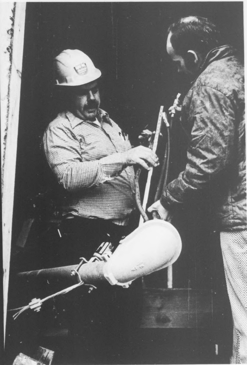
On-the-job consultation about new materials and proper techniques speeds the wiring of a new home.
