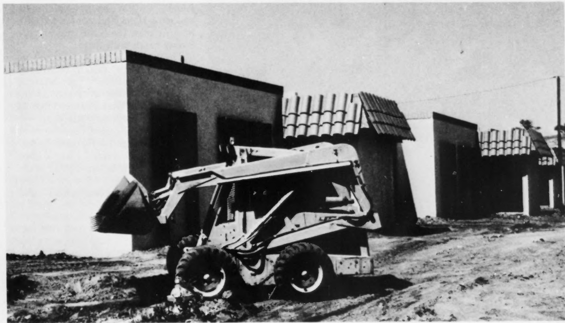
The United Church Village is the new 46-unit senior citizen complex under construction.
