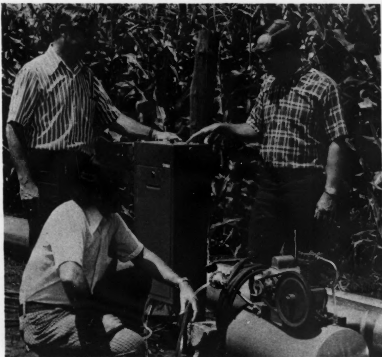
The control center for the automatic irrigation system on the Ed Thieszen farm near Henderson, Nebraska, saves labor and water. Shown checking out the center are Floyd Marsh (kneeling), general manager of the Upper Big Blue Natural Resources District; Harry Hecht, York County Extension agent (left); and Thieszen.
