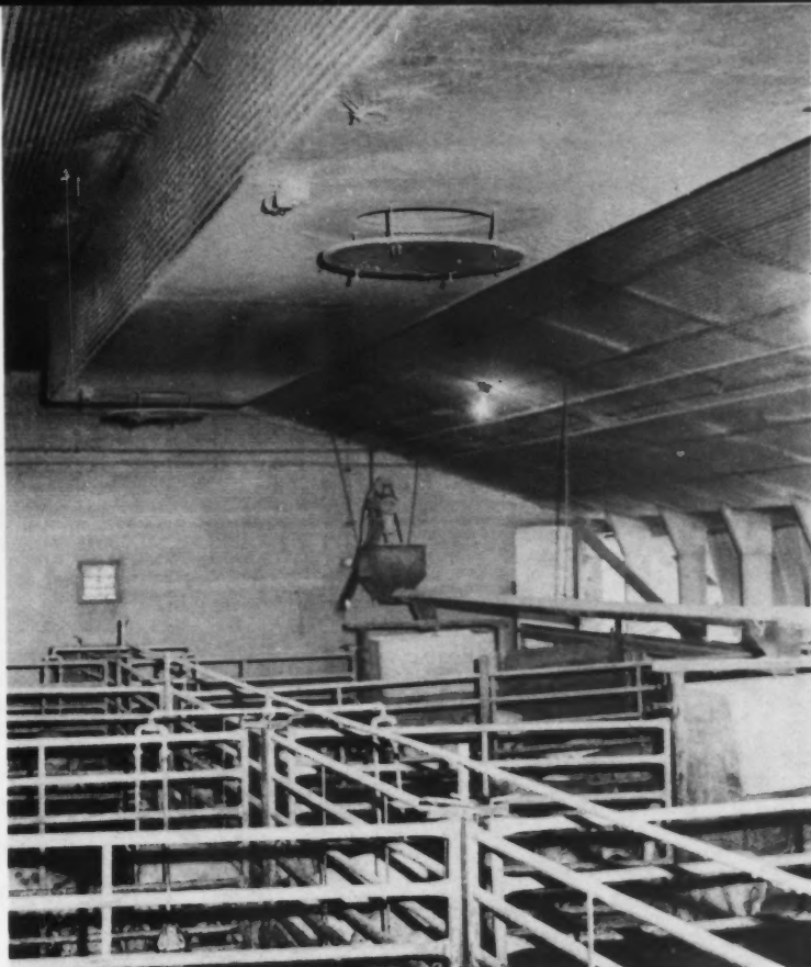
Fans pull outside air into openings at each end of the structure. The air picks up solar heat absorbed by the roofing. Fans located in the duct openings, pictured above, then blow the heated air into the building.
