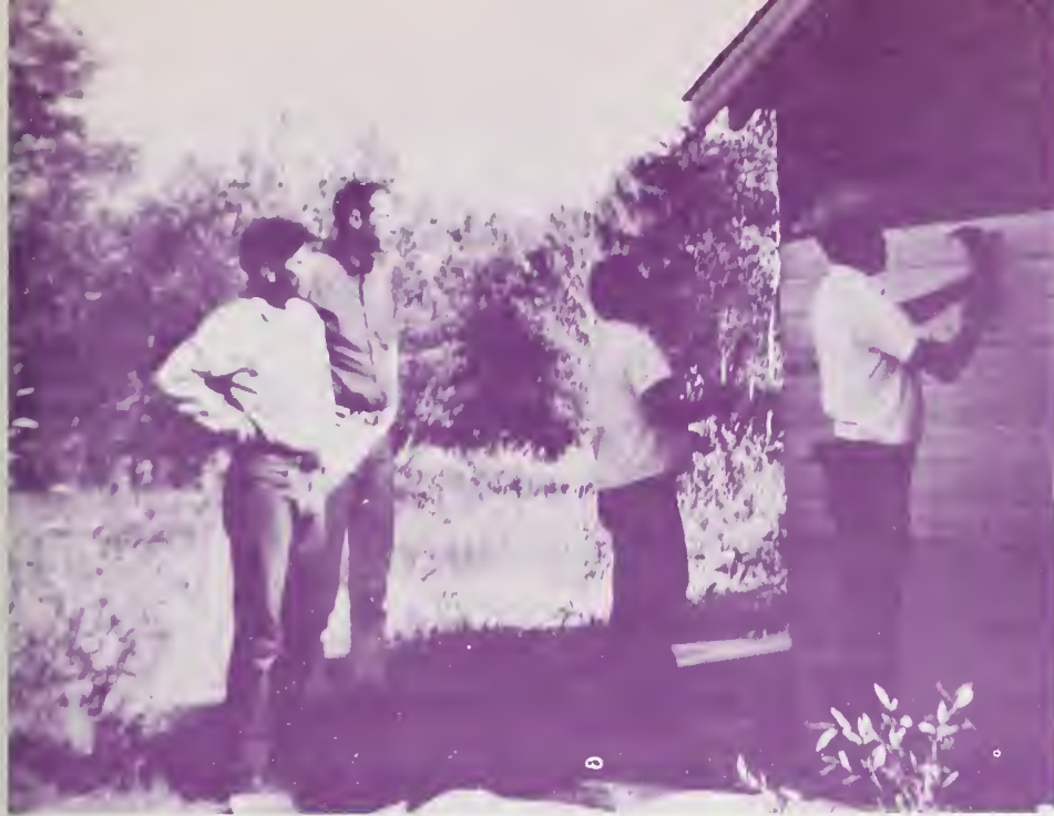
As the agent supervises, the men apply siding to the structure built during the 3-day self-help housing workshop.
