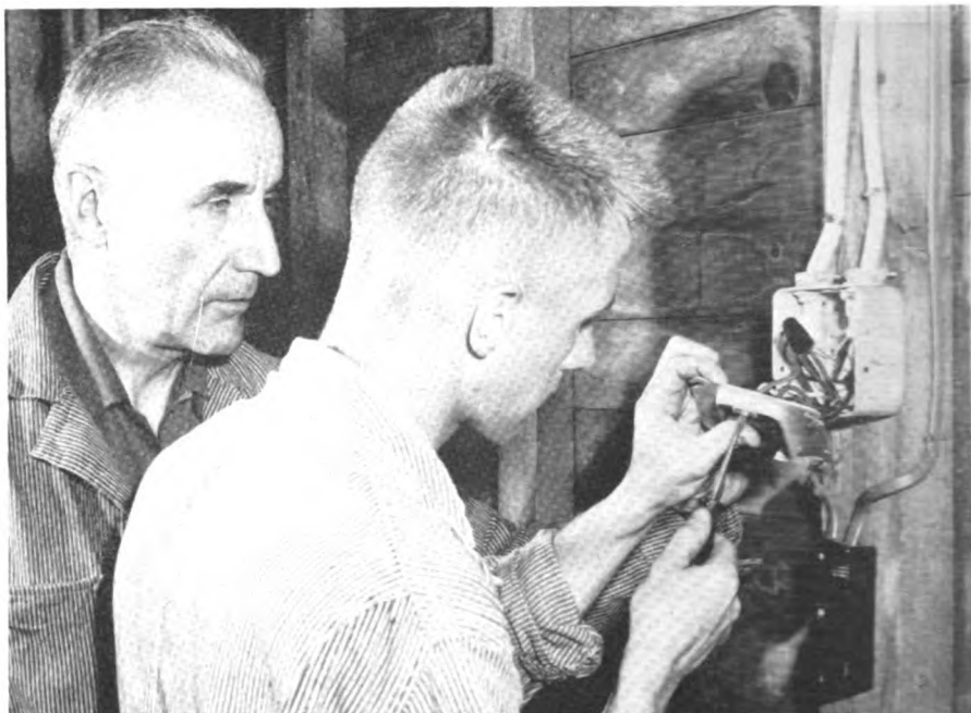
Power company representative, who earlier explained the wiring details, watches this 4-H'er apply the information.
