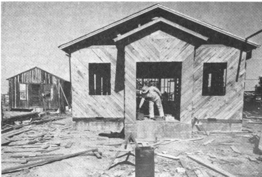
When materials for new church didn't meet specifications of new county building code, 35 members raised enough money to begin again. At left is the old place of worship.
