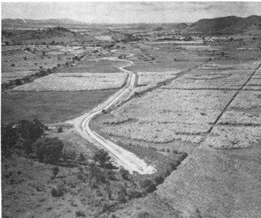
Main irrigation channel of the Lajas Valley Irrigation Project under construction by the Commonwealth Government.
