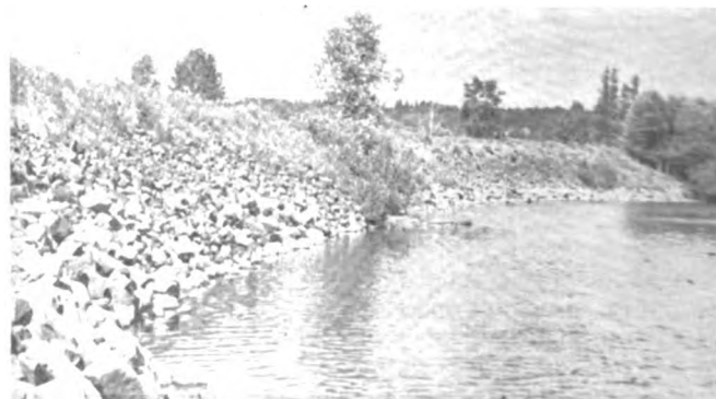
Rock ripraps, brush mats, revetments, jetties, and bulkheads are built along Washington river banks.
