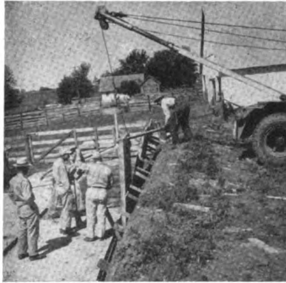
A wrecker truck is used in tilting concrete walls into place for this silo.
