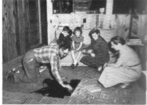
Laying a new floor attracts W. F. Gerard's entire family plus the Boone County home agent. Her followup visit is a necessary element in farm and home development to help complete plans.
