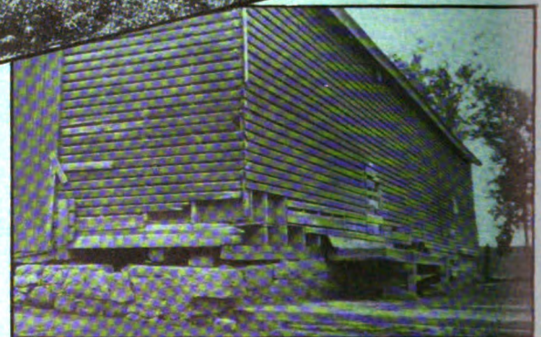
Timely repairs would have prevented this condition.
