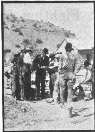
The county agent assists in threading pipe for the community well at Sena.
