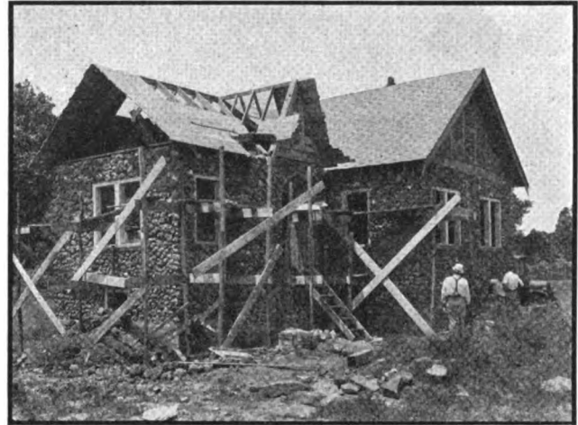
A Missouri farm home being constructed of native stones according to plans obtained through the county extension office.
