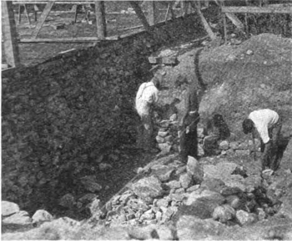
Laying the cellar wall. More than 20 tons of concrete and 150 tons of rock and gravel went into the foundation. All the work of hauling and mixing was done by the older club boys.
