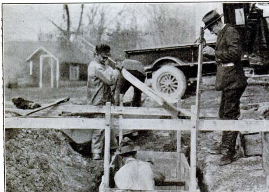
One of the community forms used for making septic tanks in Pennsylvania counties
